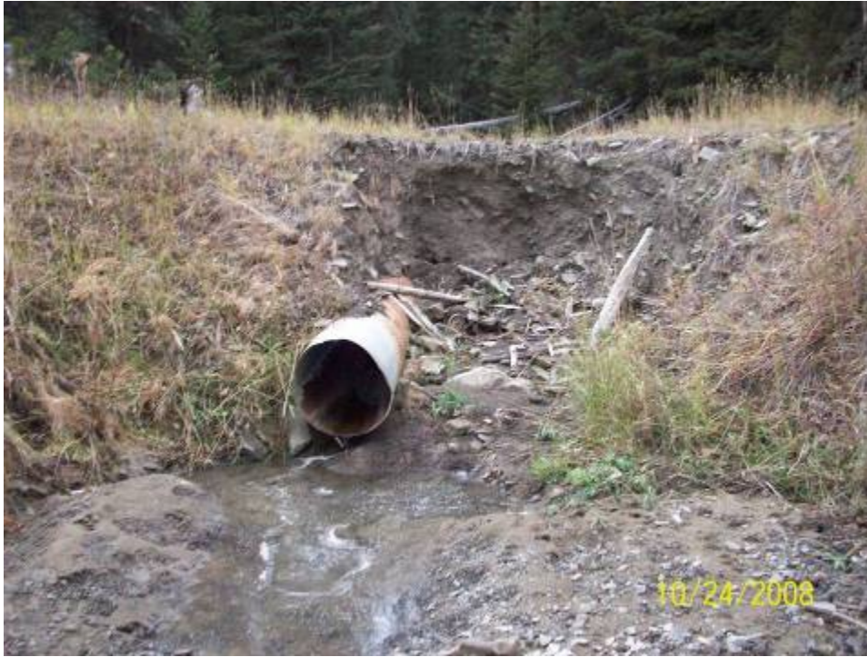
Erosion of road fill material adjacent to perched corrugated steel culvert.
