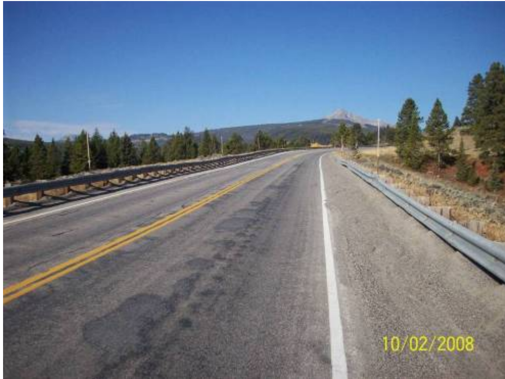
Figure F-3. Typical build up of traction sand adjacent to a guardrail along Hwy 64. Crossing C12, North Fork West Fork Gallatin River.
