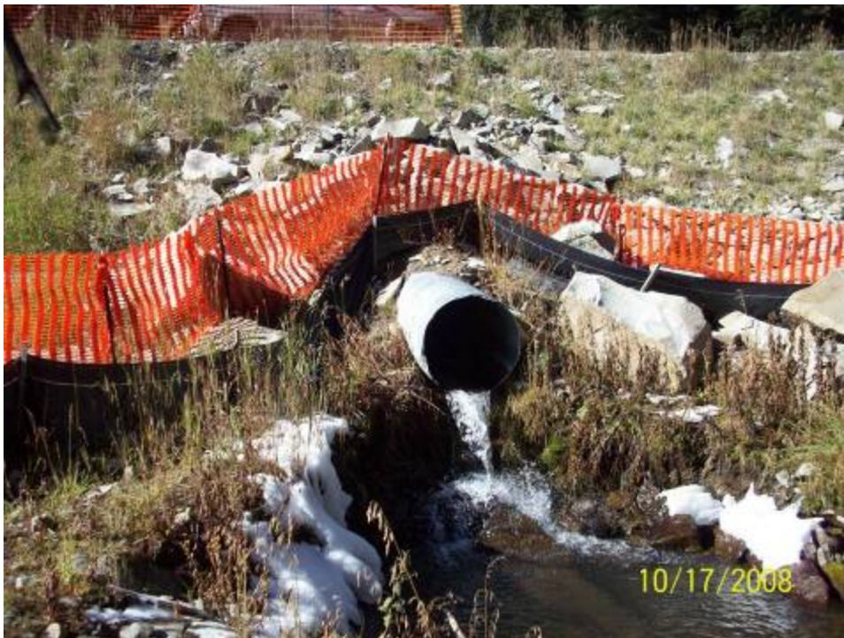
Perched corrugated steel culvert.
