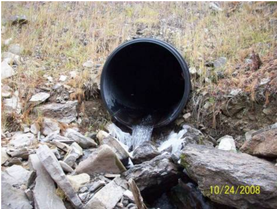
Corrugated plastic culvert, fish passage barrier.
